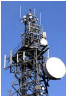
Typical Communications Hardware on Mast
